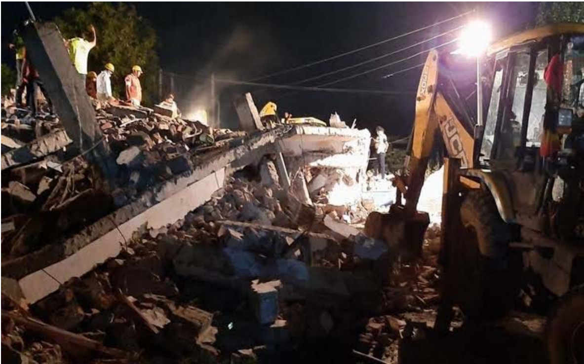
Plate 5: The Building collapse near Bukuru Mini Stadium, Jos South, Plateau State).
