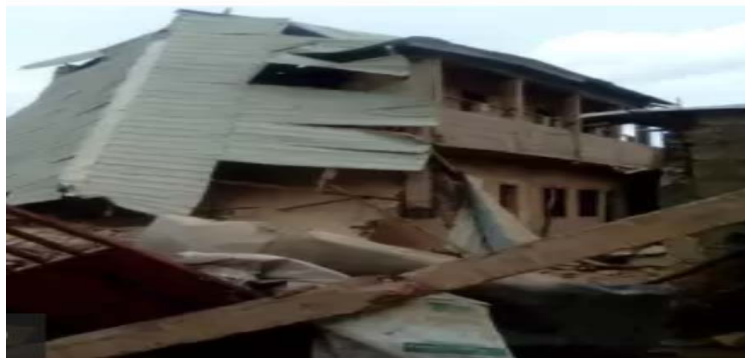
Plate 1: The Partially Collapsed Building (Job, et al, 2016).
