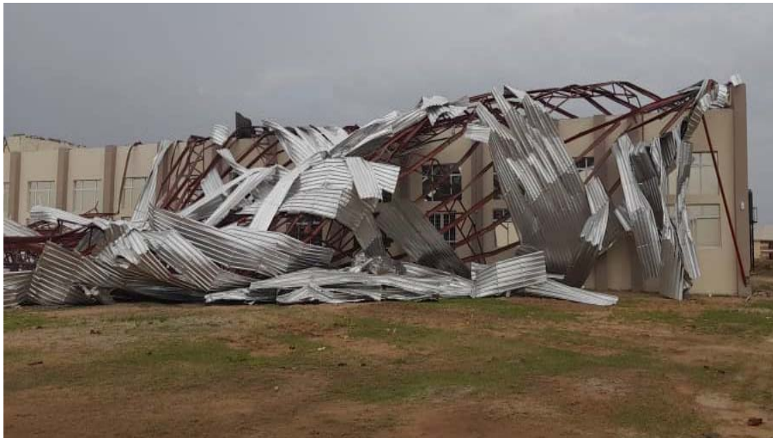
Plate 4: Blown off roof of the Indoor Taekwondo Gymnasium. Source: https://www.unijos.edu.ng/WindstormWreaksHavocinUnijos
