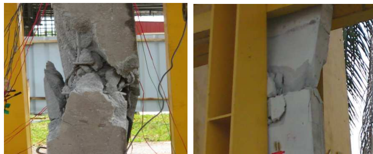
Figure 7: Crack and crush at mid-height of panel PA-12
