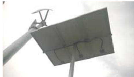
Figure 1: Hybrid System: - Vertical Axis Wind Turbine & 3 Solar Panels In Yong Peng, Johor
