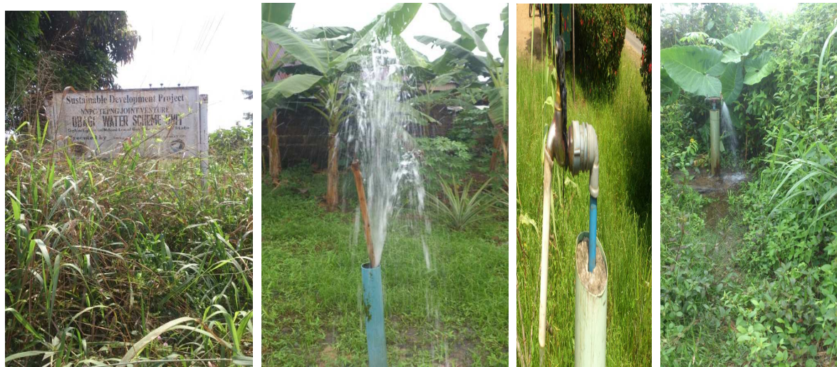
Fig 8: Water wastage from ill-maintained water facilities as donated by TEPNG to Egi communities
