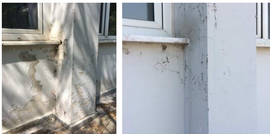
Figure 10: Wall Deteriorations Most Likely Originating From on Lack of Insulation and Moisture Ingress
