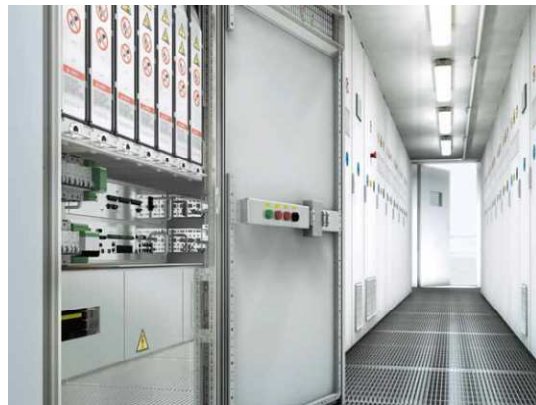
Figure 11: Siestorage: Battery energy storage system for a sustainable energy supply
