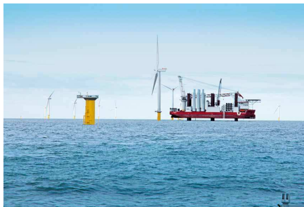
Figure 14: Installation of wind turbines (SWT-3.6-120) at London Array offshore wind power plant. The goal is to produce 18,000 MW by 2020.
