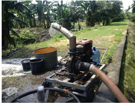
Figure 5. Pump used for the testing on the different blends of biodiesel
