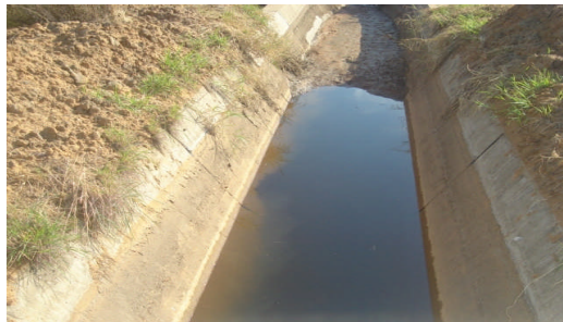
PLATE 1: SECONDARY CANAL FILLED WITH SILTS DOWN STREAM
